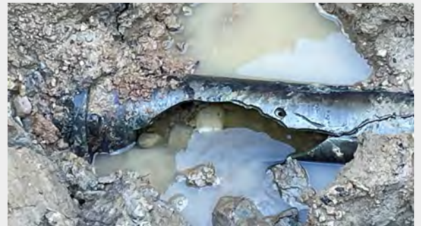
Pictured: Water main break that occurred on Johnson & Harding Street.
